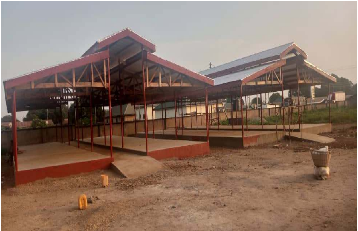
2NO. 40UNIT MARKET SHEDS COMPLETED AT KPASA NEW MARKET FOR 'COCOA ASE' TRADERS
